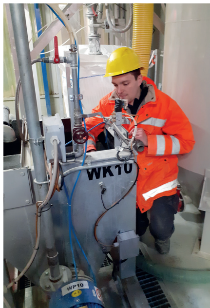
▲ Pic 3 Checking the flow of raw materials.
